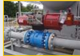
Hydraulics and Instrumentation
